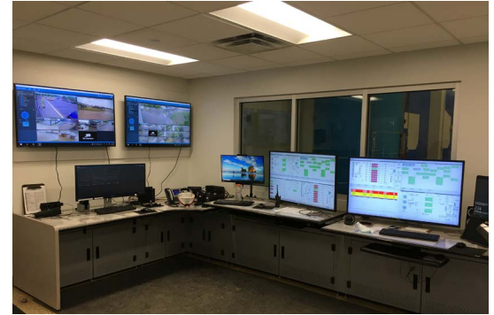
East Plant control room
